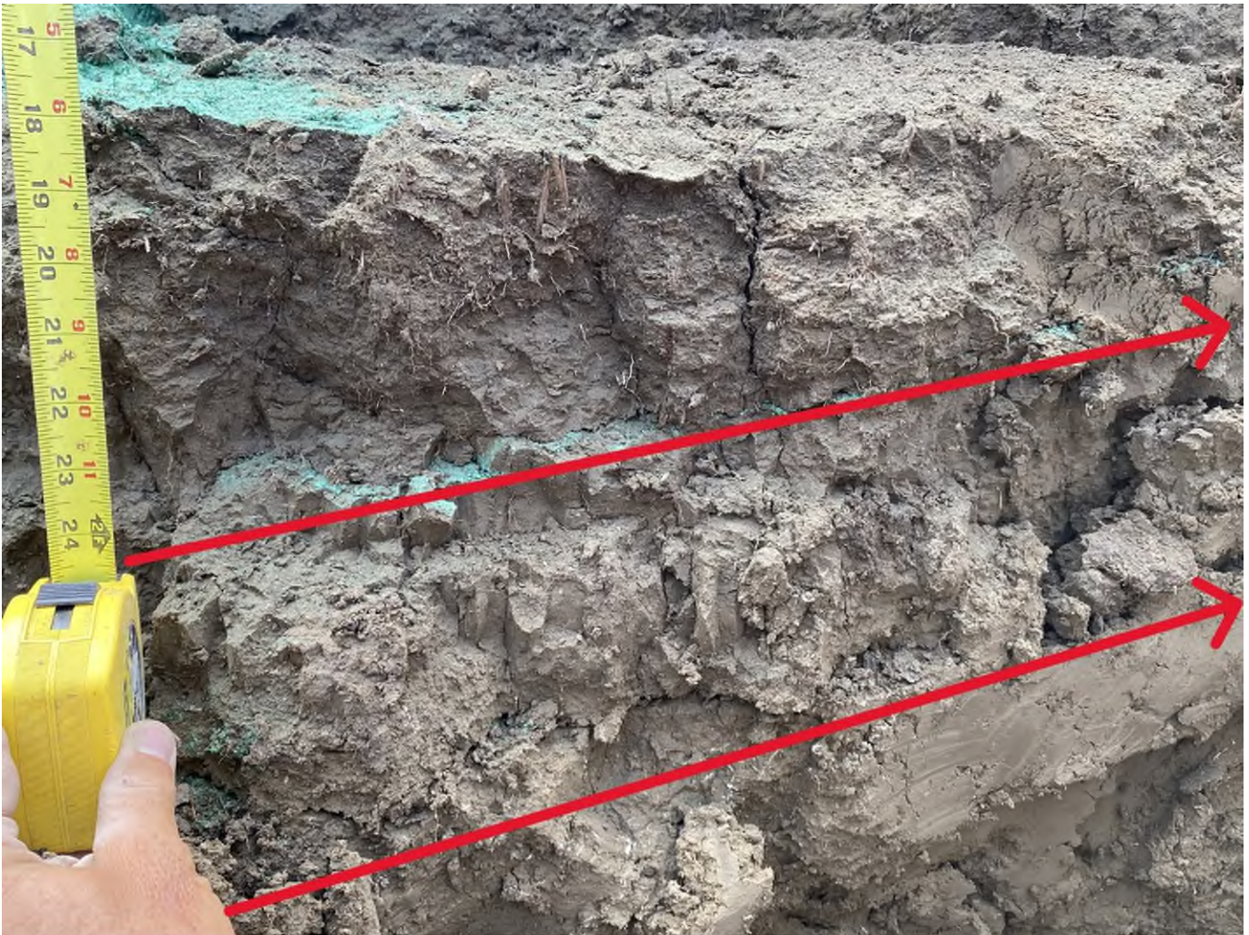
Image C-4: Test #2 - Upward Horizontal Fracture @ 24" & 31" Deep with Mica Trace Along Surface of Fracture
